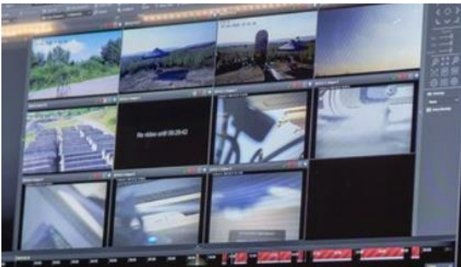
(6b) – Scada Station (6c) – Scada Video
